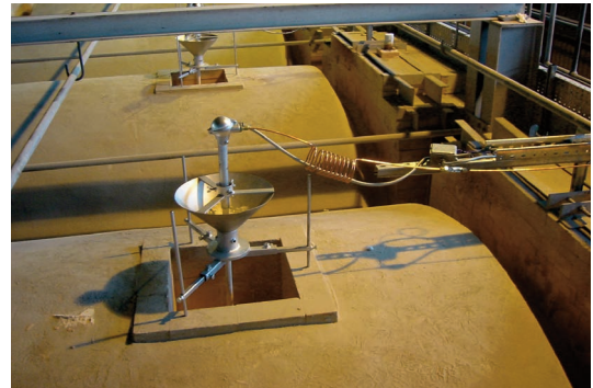
Oxygen sensors installed on regenerator crown at a crossfired furnace
