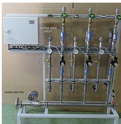
Cooling water control skid
